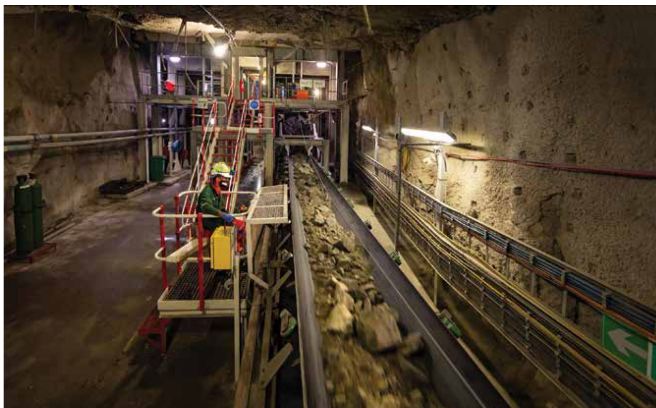
Bottom of Silo 2 discharge on 708 level – measuring flask feed conveyor at Styldrift
