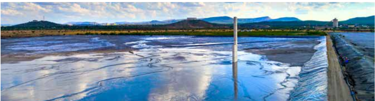
The newly expanded Maseve tailings storage facility (TSF). To prevent seepage the walls and base are lined with 1.5mm thick HDPE geomembrane liner
