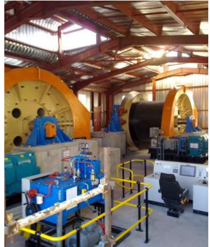
Main & Service Shafts Stage Winders:
