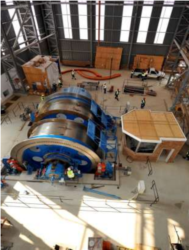
Main Shaft Personnel and Material Winder (5.5m D):
