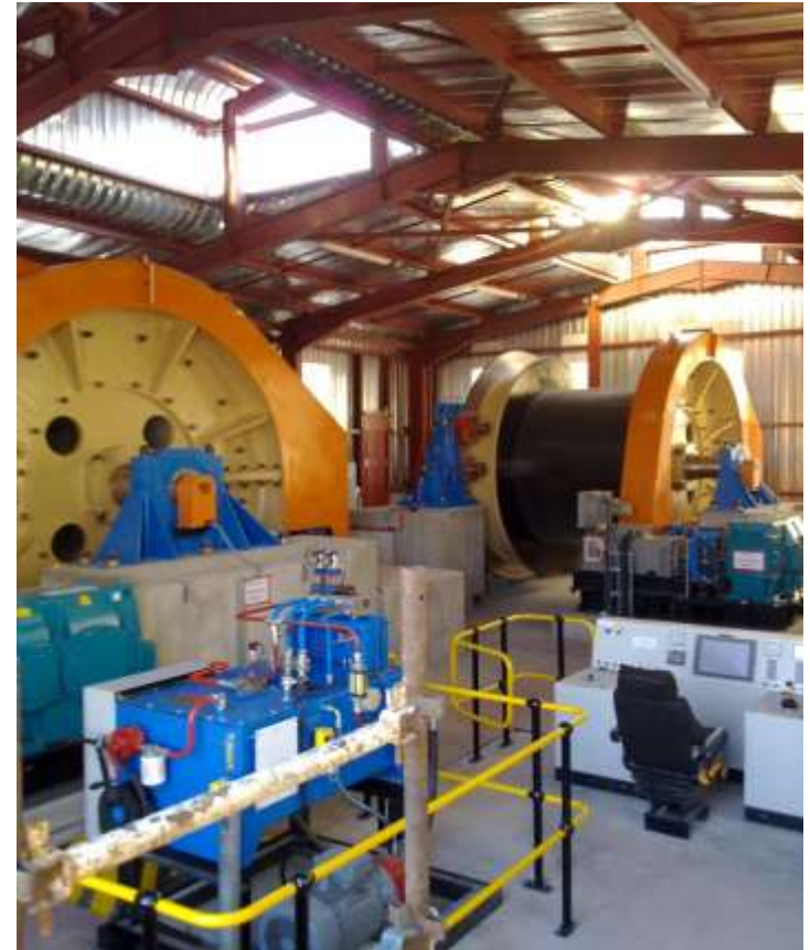
Main & Service Shafts Stage Winders:
