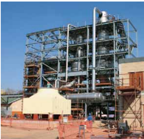
Construction in progress at the crystalliser, which will ensure that Refineries complies with zero effluent once the current expansion project is completed.
