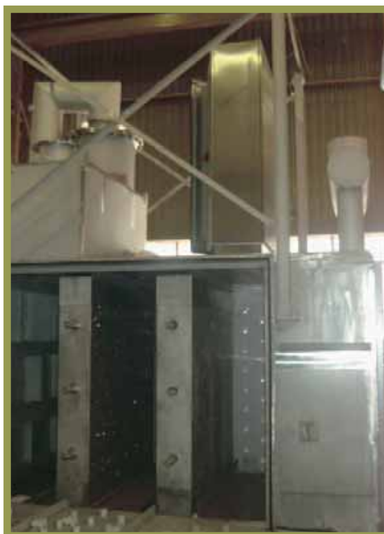
One of the ultra-violet reactors installed at Refineries.
