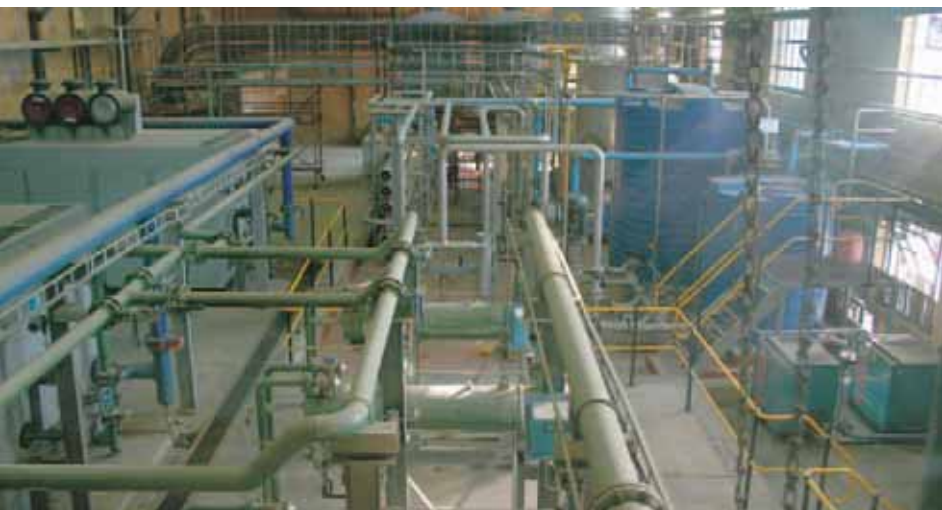
The new Effluent Treatment Plant at Refineries.
