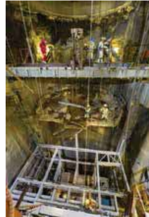
View of shaft loading box construction activities taking place between 708L and shaft bottom at Styldrift I Main shaft
